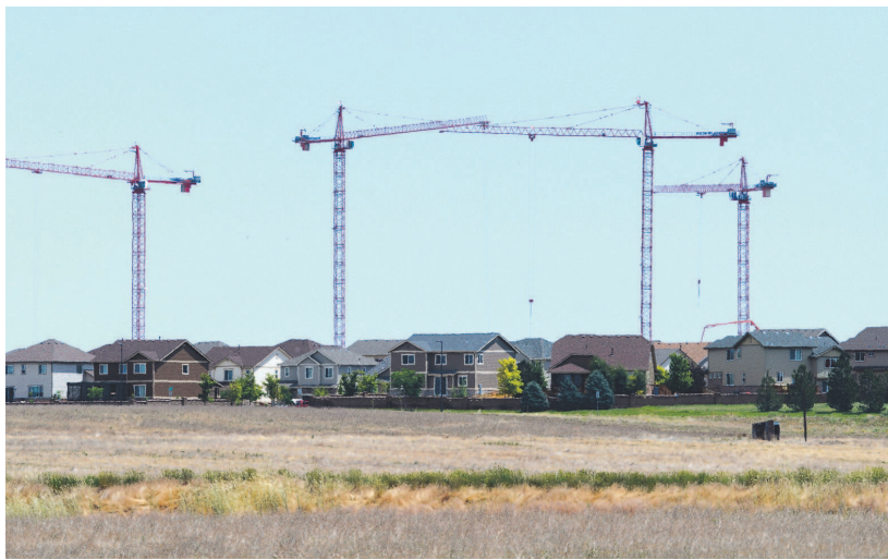
Gaylord Rockies Resort and Convention Center construction cranes behind a housing development. Andy Cross, The Denver Post
